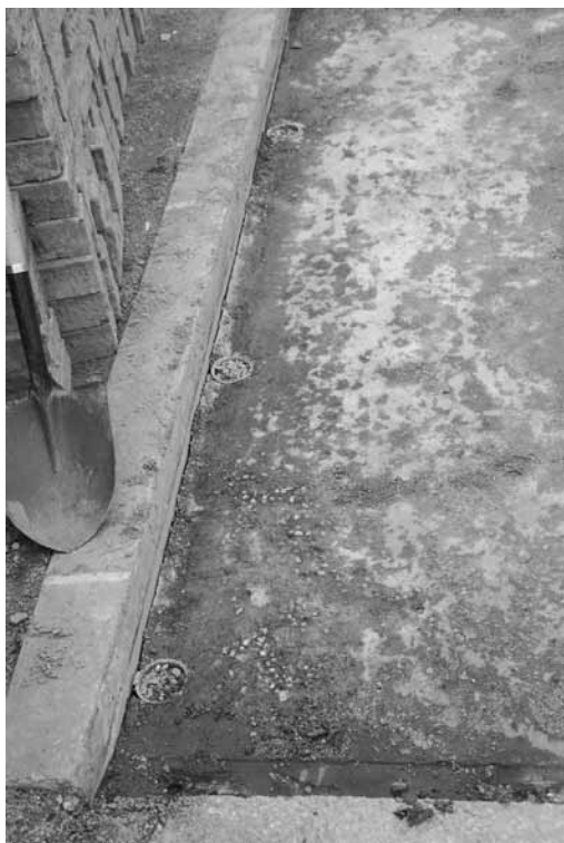
Figure 5-5. Drain holes placed at the lowest elevation in an asphalt pavement to be overlaid with concrete pavers.
