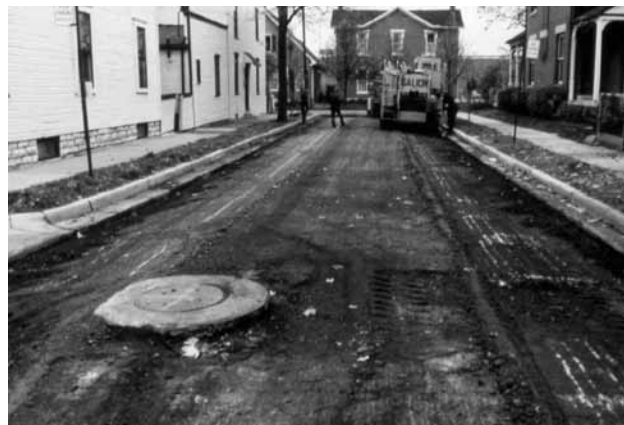
Figures 5-3 and 5-4. A milling machine can create a crown (or flatten one) in a street, thereby adjusting the grades for better drainage.
